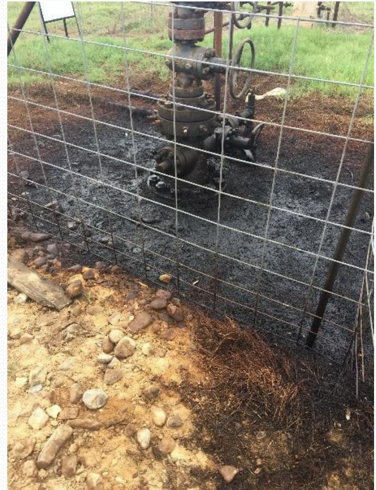
Additional Ground Work Is Needed to Remove the Stains
